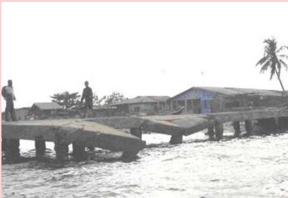
A damaged jetty in one of the riverine areas of Lagos State
